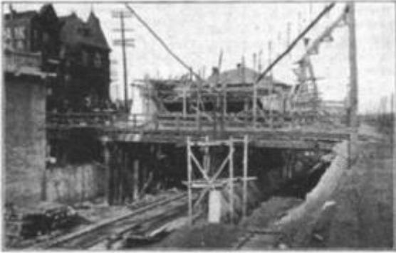
Construction View. Temporary Crossing of Street Car Tracks Over Missouri Pacific Westbound Tracks and at Grade with Missouri Pacific Eastbound Track
